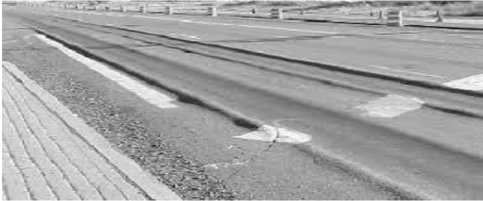
Figure 4 Photo demonstrating an example of asphalt layer rutting [38]
