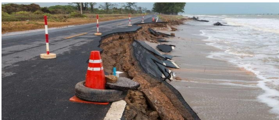
Figure 7 Coastal road eroded by waves due to sea level rise [47]
