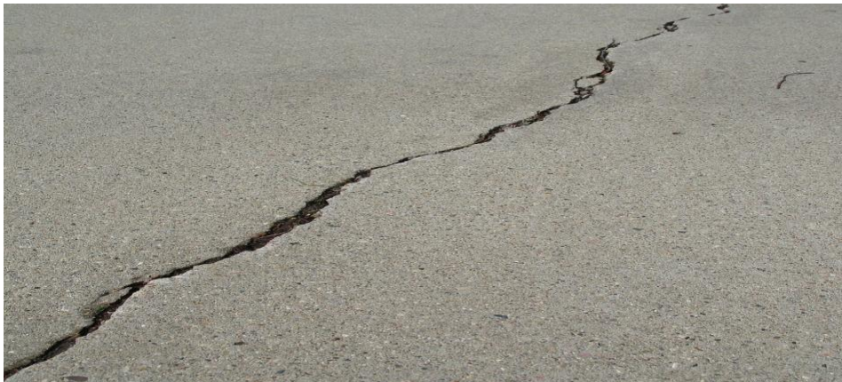
Figure 10 Shrinkage-induced pavement cracking [56]
